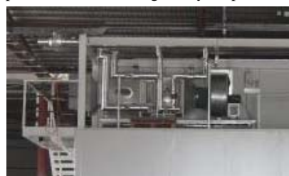
Air cooling and filtering facilities
