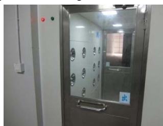
Air shower room
