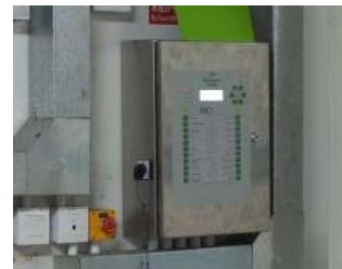
Display panels outside the mushroom cultivation room showing different indices and the operation of facilities
