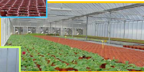
Large ventilating fans enhance the air ventilation.
