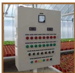
A control panel of the environmental control devices
