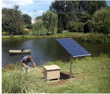
Use of renewable energy
