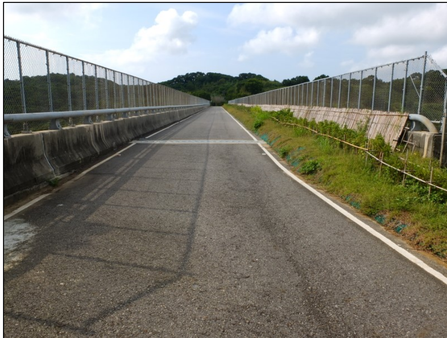
Figure 3. Animal passage constructed on an existing vehicular bridge in Taiwan (Academia Sinica Center for Digital Cultures, 2018)
